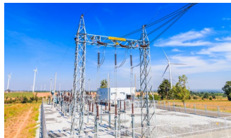
Substation partial discharge
